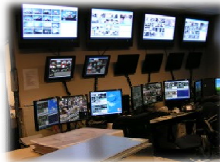
Central Surveillance Data center
